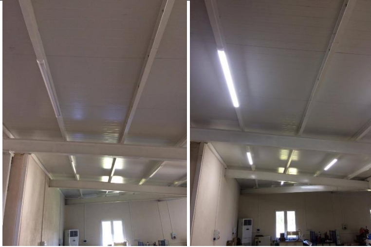
Example of Energy Efficient Appliances Usage: University is replacing the conventional lamps with LEDs
